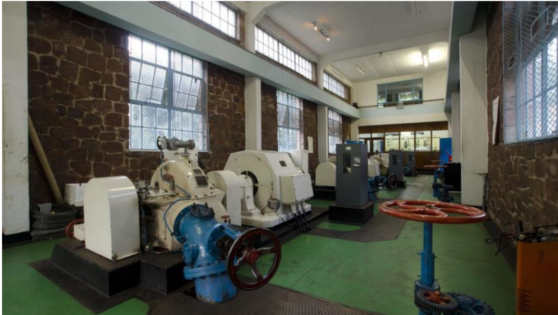
Figure 8: Small hydropower station on Lake Tanganyika in Zambia. 51
