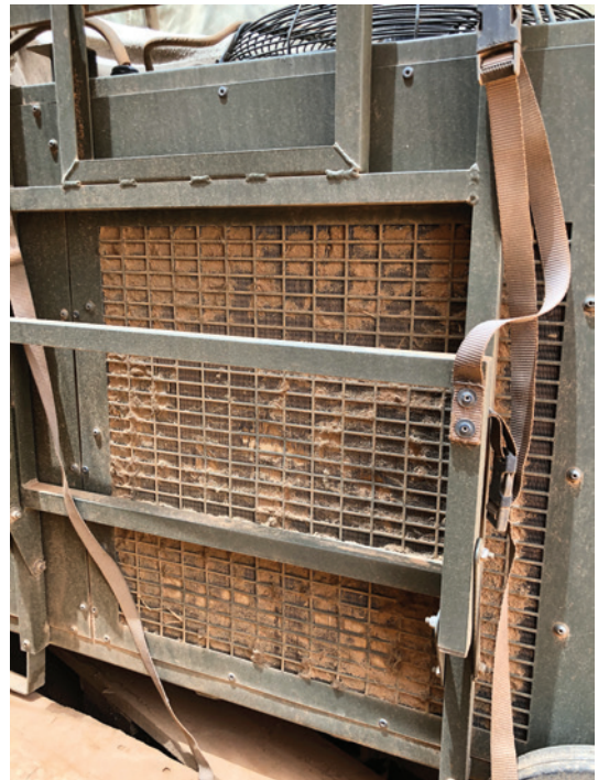
Figure G1: Example of a Dirty Air Conditioning Coil Providing Discomfort
