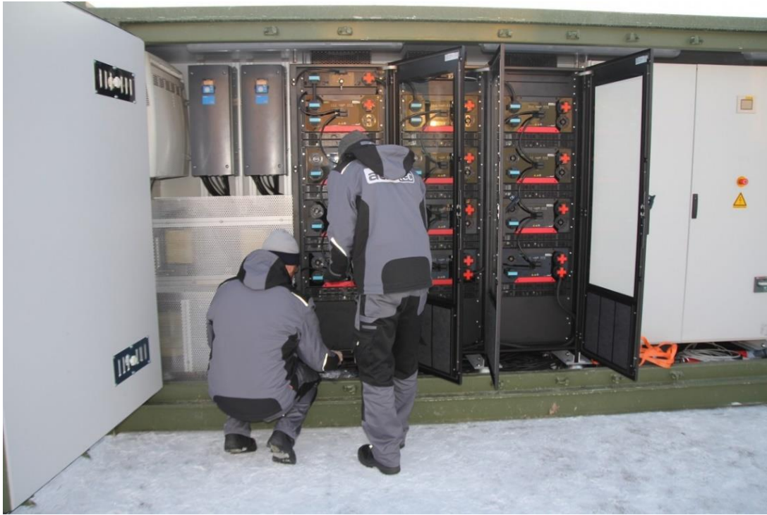
Figure 16. Access of maintenance and other local personnel to EMS and associated equipment requires strict control
