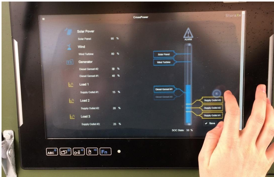
Figure 15. Photo of a control panel for a wind power system that can be connected to the EMS of a smart grid in a camp. The HMI is software that presents information about operations and easy access to the devices monitoring and controlling the equipment. Unauthorized access to this panel for malicious purposes or human operator error can lead to service disruptions of damaged equipment.
