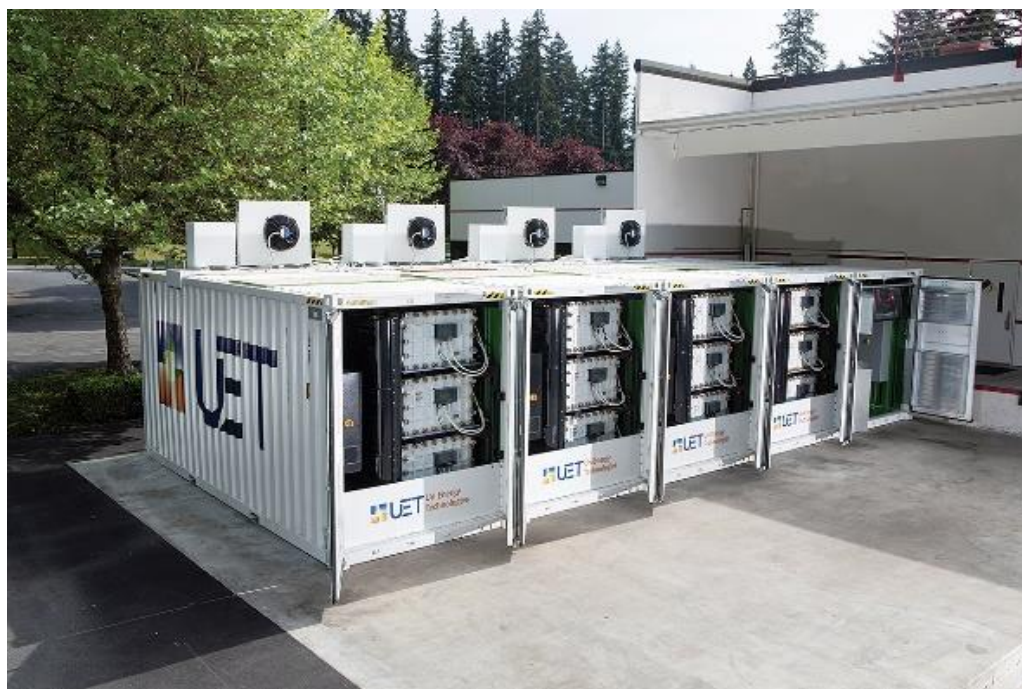
Figure 5. RFB stacks housed in a container like enclosure 33 .
