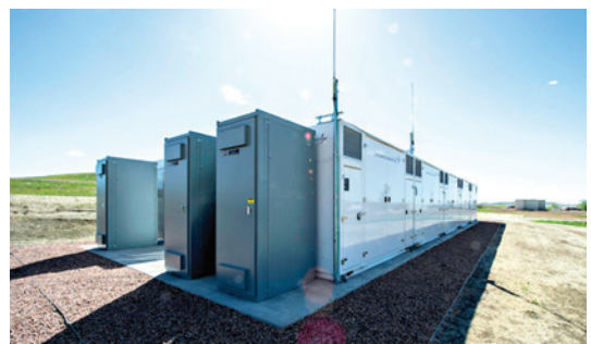
Figure 12: Utility scale lithium-ion Battery Energy Storage System (BESS) installation at Fort Carson, USA
