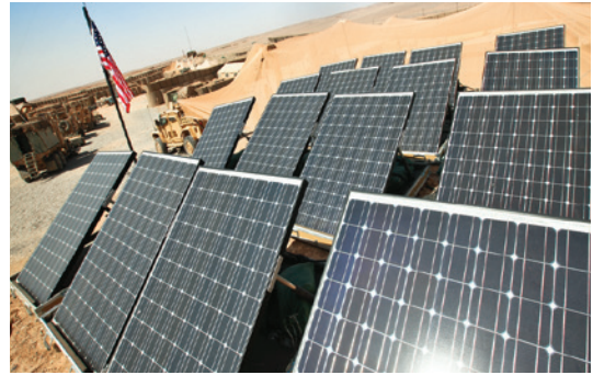
Figure 8: Solar panels at Patrol Base Boldak, Helmand province, Afghanistan
