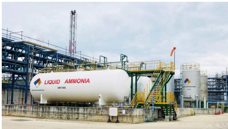
Figure 7: Ammonia storage facility in Japan (Harding 2020).
