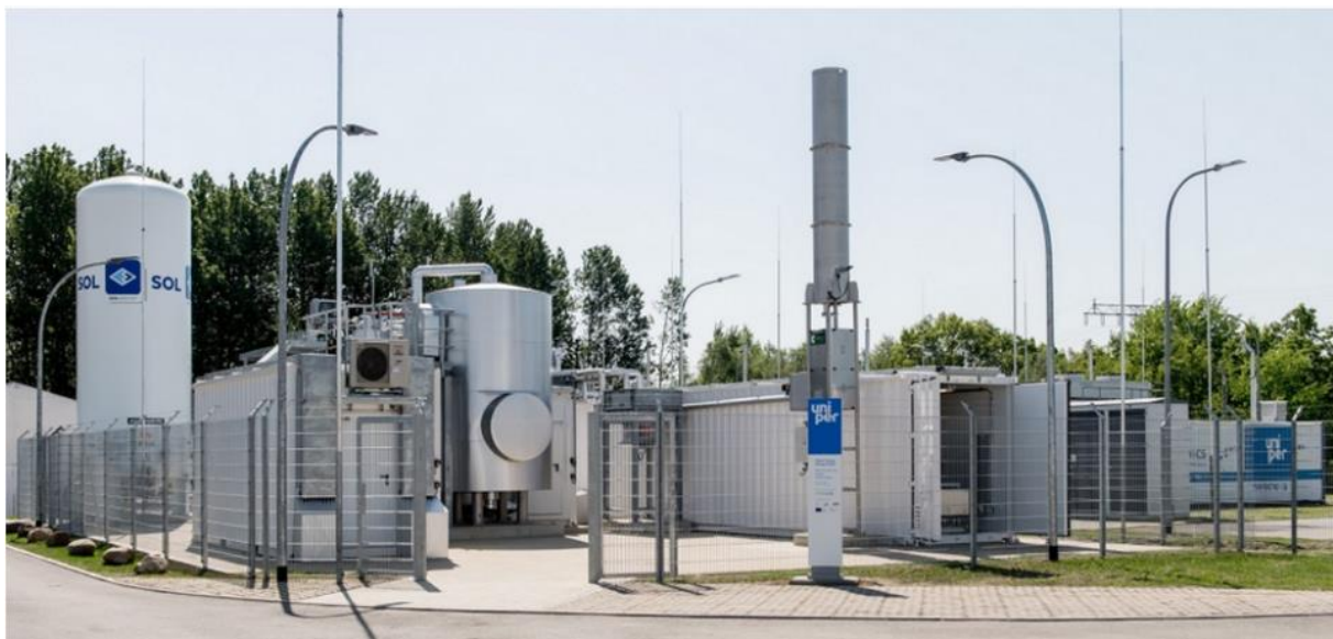
Figure 10: The Power-to-Gas Plant Falkenhagen in Brandenburg, Germany is operated by Uniper SE since 2012. Uniper was outsourced in 2015/2016 from e.on AG, one of the former regional monopolists for electric power generation in Germany. The two containers on the right hand side of the picture hold the electrolysers. The left hand side shows the methanation unit for conversion of carbon dioxide (CO 2 ) into methane (CH 4 ) 24 .
