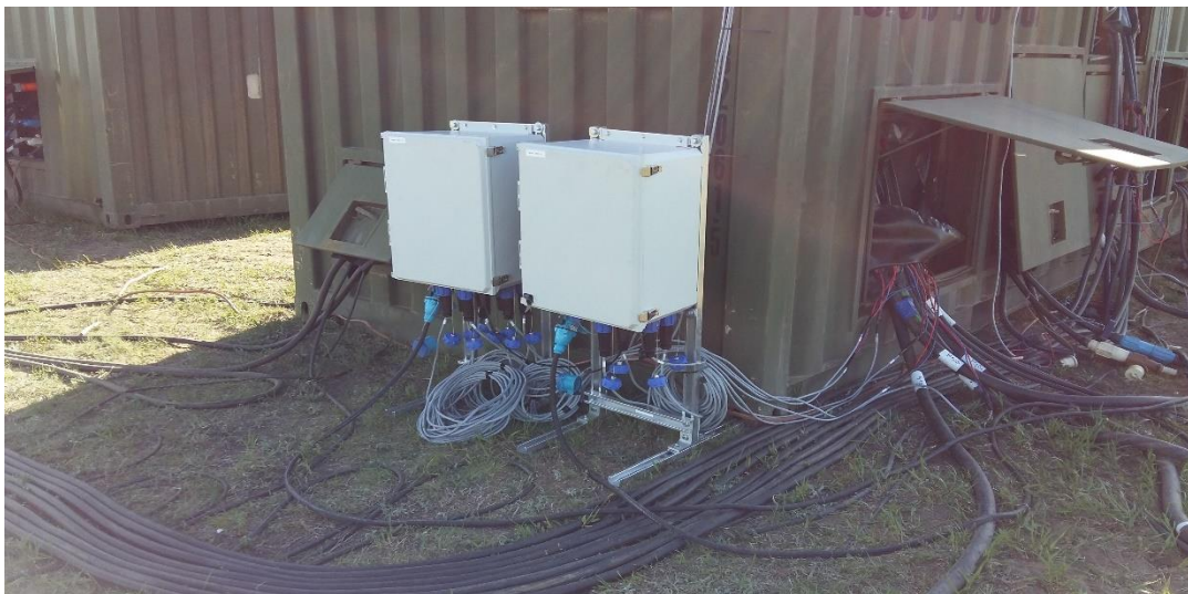
Figure 2 - Non-Intrusive Electrical Meters Installed at EXERCISE MAPLE RESOLVE 2017 (Wainwright, Alberta, Canada)
