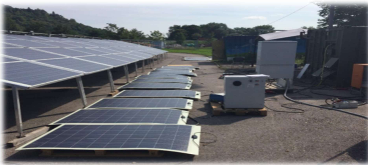
Figure 21. Part of additional 4Kwp solar panel array (Pfisterer, 2017)
