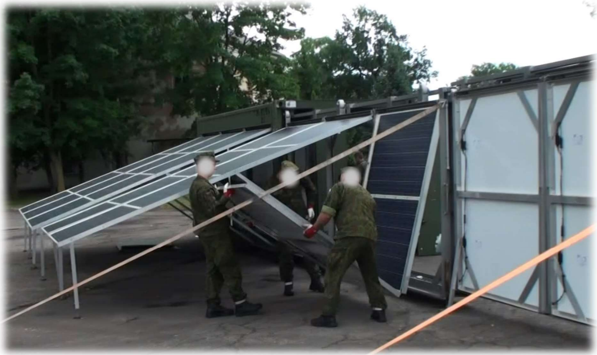
Figure 22. Solar panels assembly, Marijampolė, Lithuania
